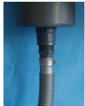
Figure 23b — Hose attached to thru wall skimmer
