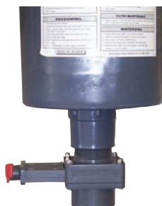
Figure 4 — Slide valve installed in bottom of skimmer
