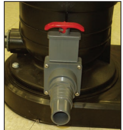
Figure 1 — Slide valve attached “TO POOL” on tank
